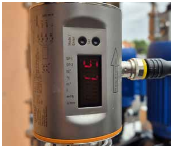
N. 1 FLOW METER FOR EACH PUMP/PRODUCT
